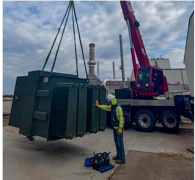
Journeyman Lineman Kyle Miller steadies a transformer that was installed at POET.
